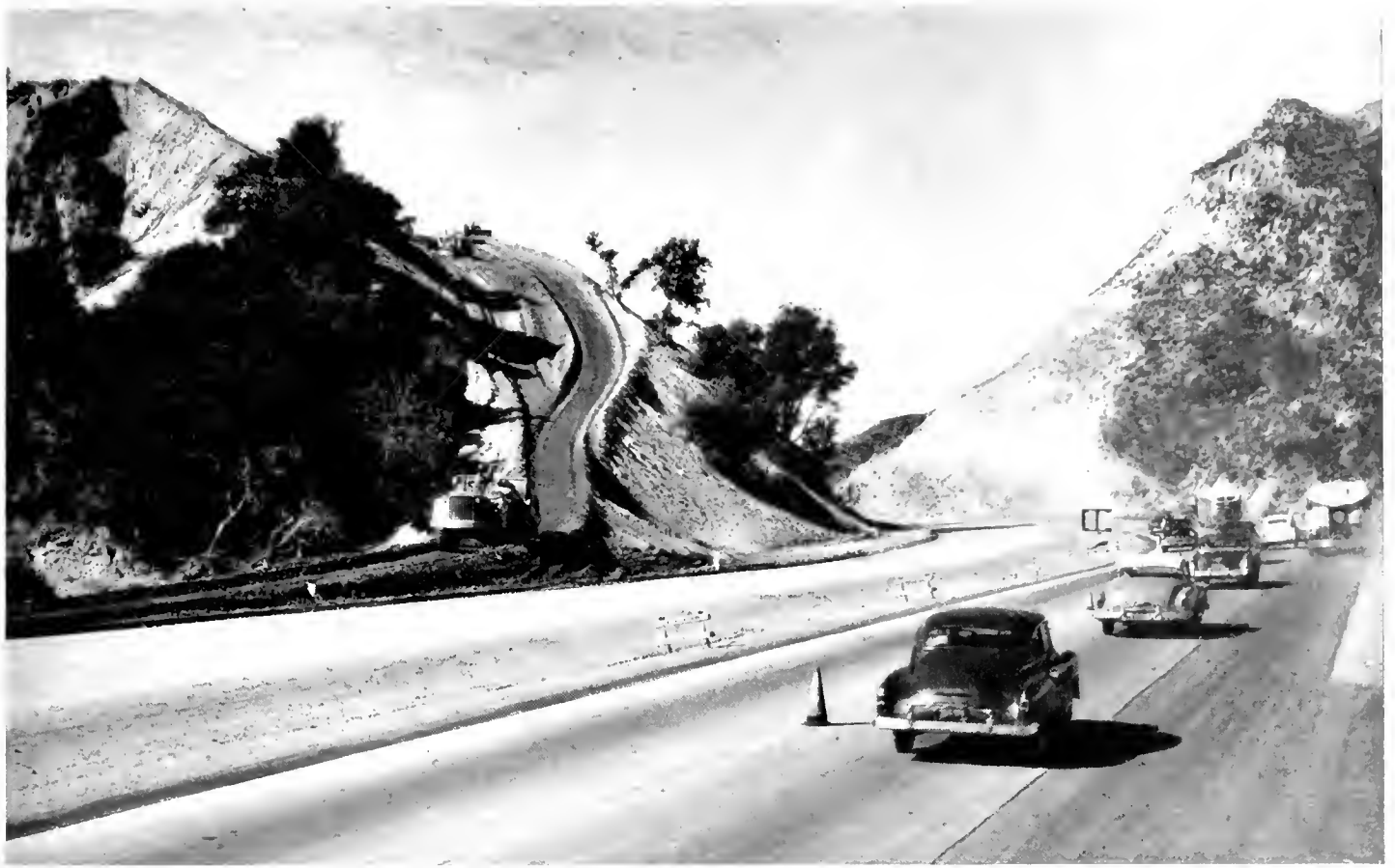
Looking northerly along completed Ridge Route section in Weldon Canyon, showing contractor's equipment descending 40 percent grade with embankment material for Weldon Canyon fill that is being obtained by widening the Weldon Canyon Summit cut
